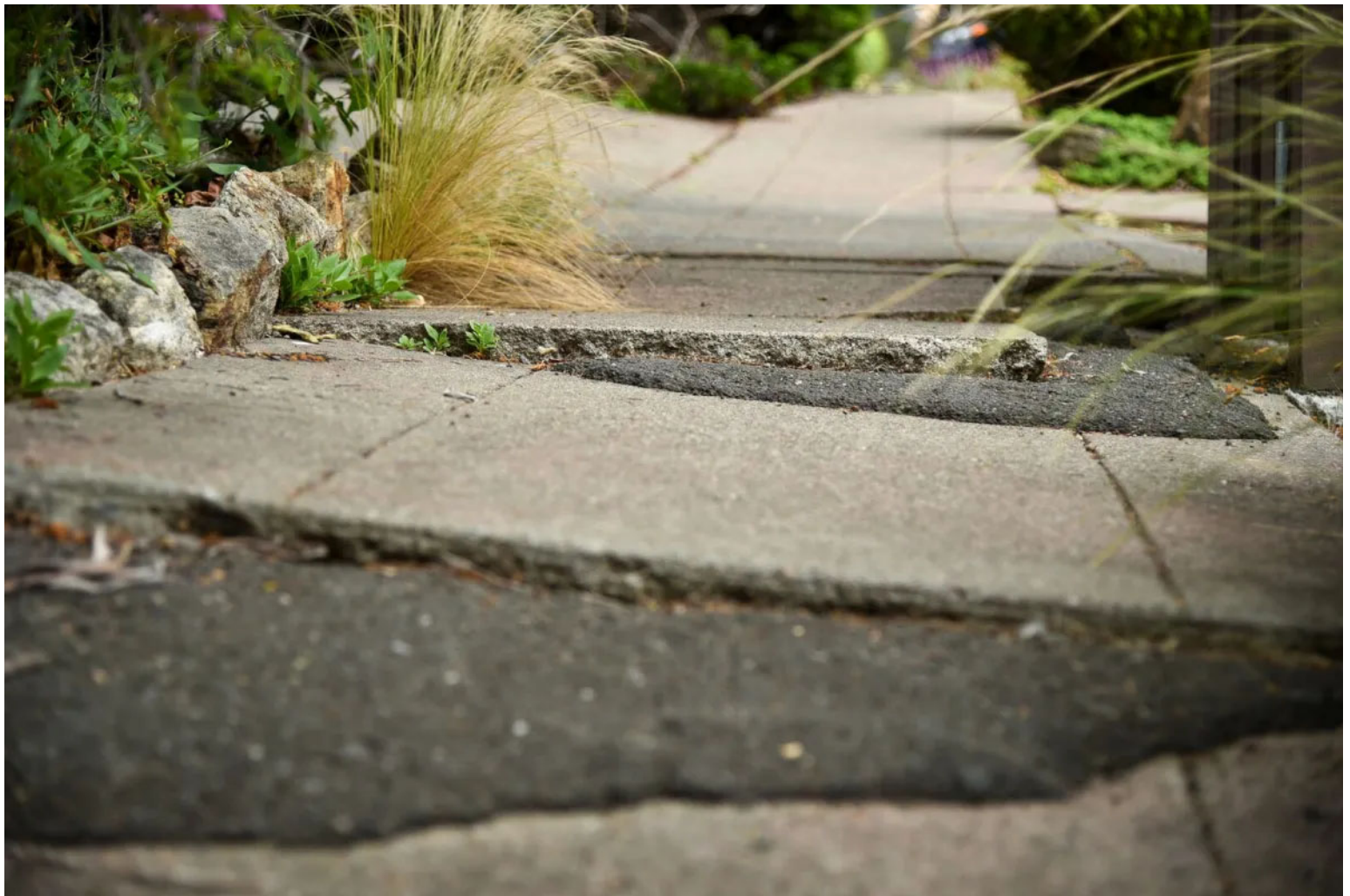
A sidewalk in need of repair in the Berkeley Hills. File photo: Jerome Paulos
